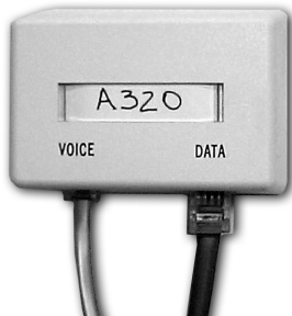
FIGURE 6-9 Properly labeled wall jack
